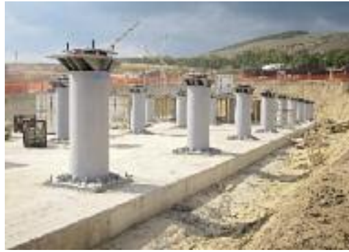
Fig. 20 Reinforcement in a foundation plate with concrete columns and steel columns with isolators on a casted plate.
